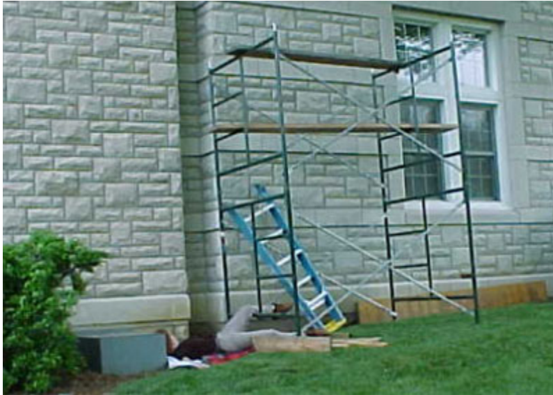
Exhibit 4. Scaffold violations contribute to worker fatality.
